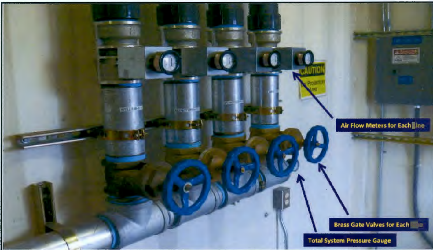
Photo 5: View of piping manifold for the four well lines.
